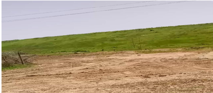
Figure 6: A Section of the downstream slope of Tiga Dam vegetated with Grass
