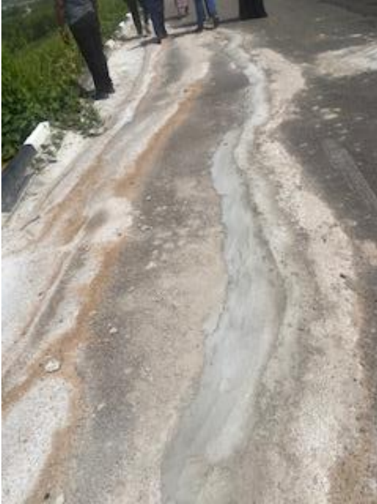
Figure 7: A section of cracks sealed by cement on the Dam Crest
